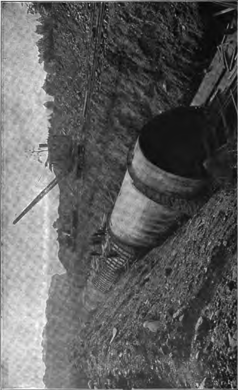
PLATE 126.—Contract 15. Steel Forms and Locomotive Crane for Building Cut-and-cover Aqueduct. Continuous method was here used, forms being used "telescoping," 60- to 75-foot section concreted daily.
